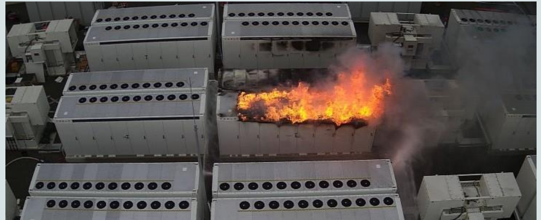
Li-ion battery burns for 3 days, “out of control” August 2021
