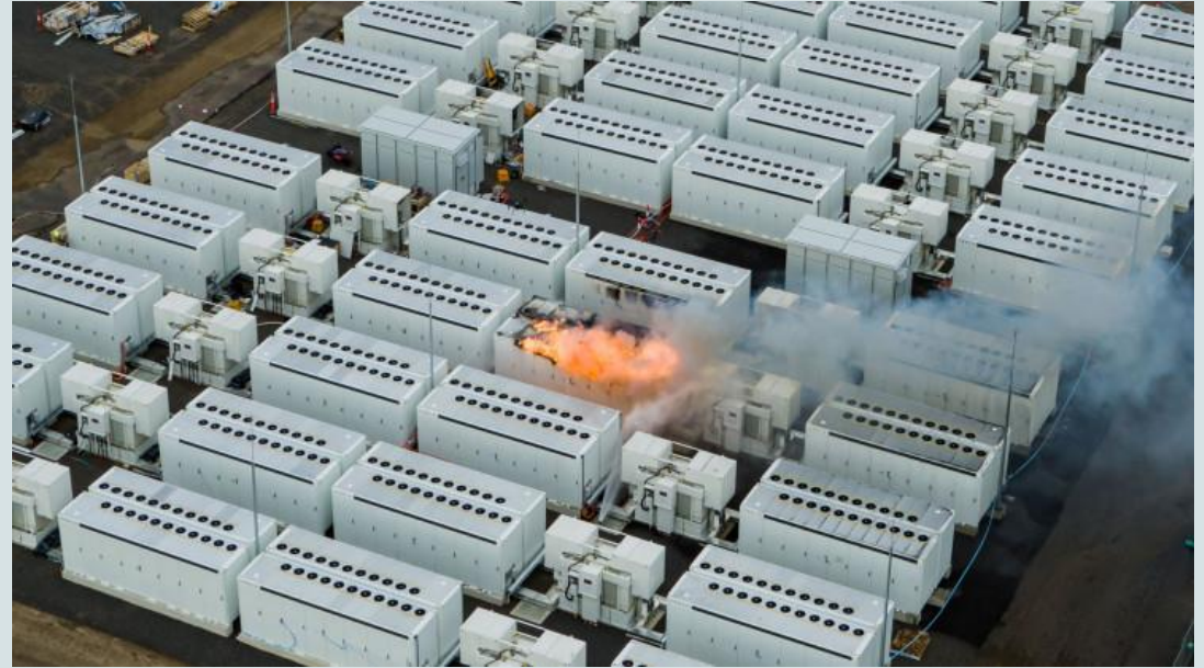
450 MWh li-ion battery, largest in southern hemisphere
