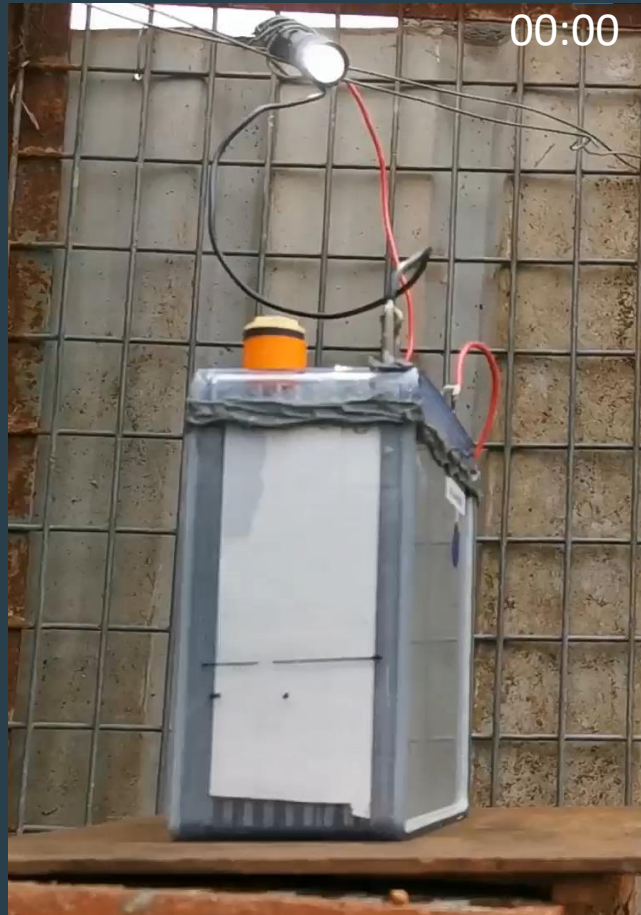
Gelion battery cell
